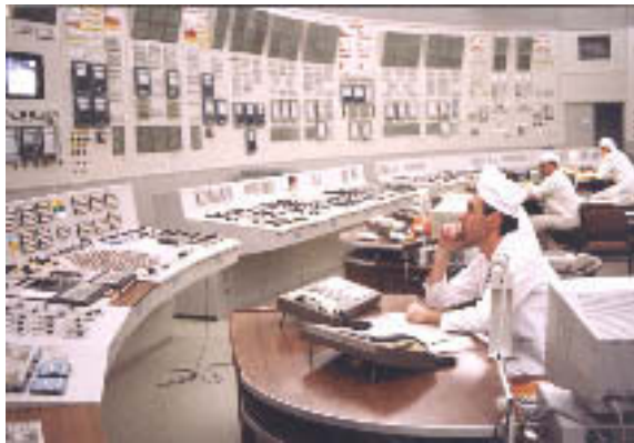
Figure 3-6 Control room of Kola NPP (Photo: NRPA)
