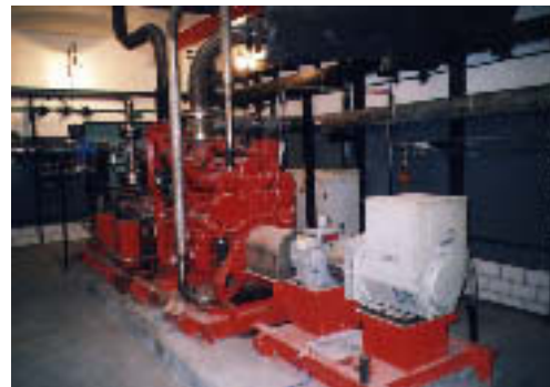
Figure 3-2 One of the diesel engines/pumps for the CEFWS at Kola NPP.(photo: Storvik)
