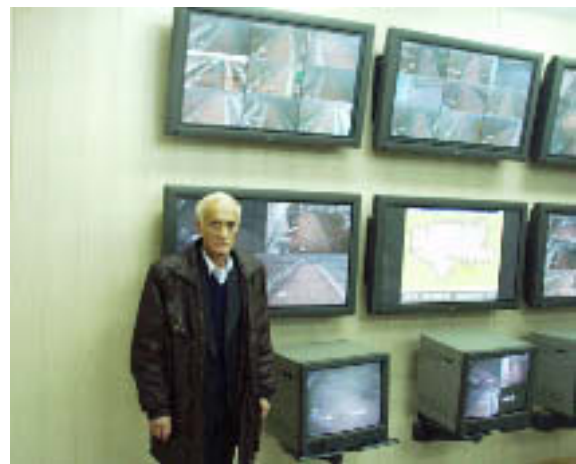
Figure 4-2: A representative of INPP (Mr. Velishkovsky) in front of the monitors for the perimeter surveillance system.
