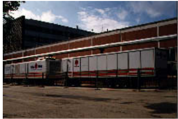
Figure 3-1: Mobile emergency power plant (Photo: NRPA)
