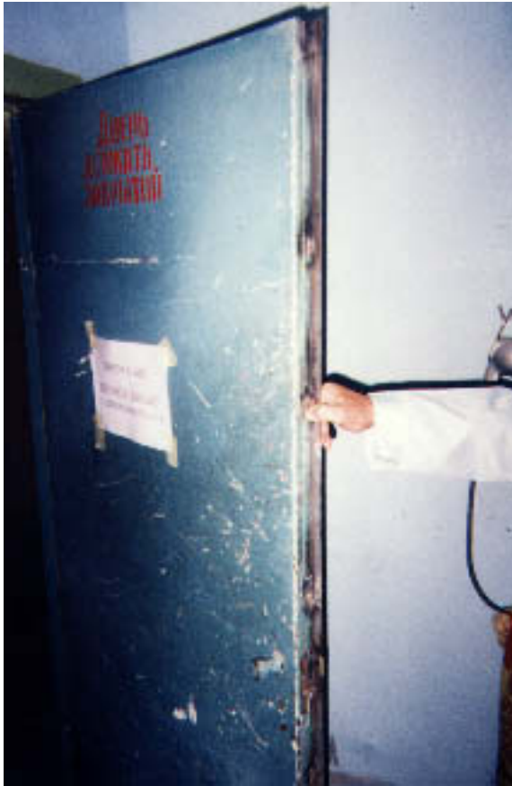
Figure 4-3: Example of a fire door to be replaced (Photo NRPA).
